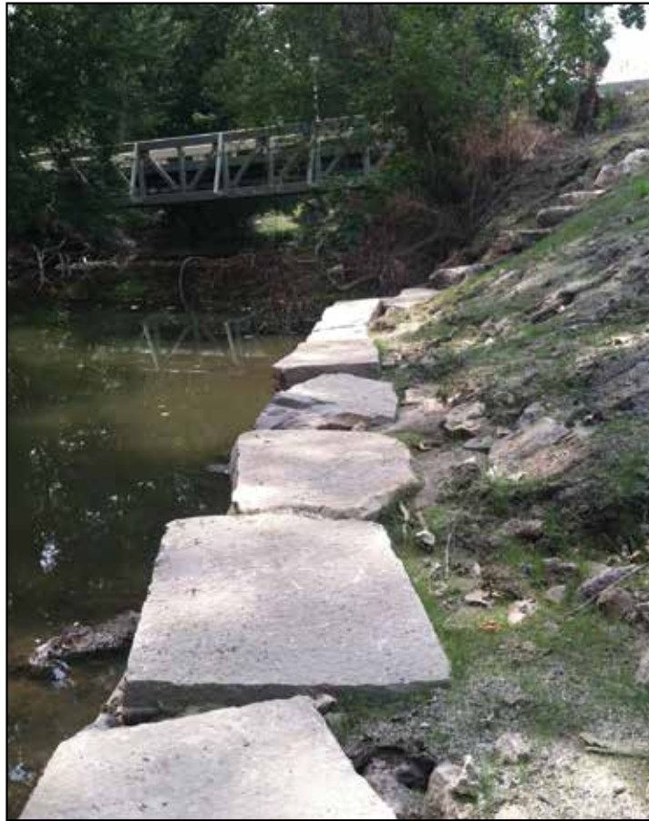
Above: LUNKERS, post construction. Below: Placement of eight foot section of LUNKER in Reach 3.
