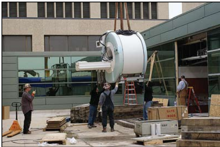
HEAVY LIFTING: Workers hoisted the MRI magnet into position. The MRI machine, which was moved in March, is now located in the Imaging Center of the UT Medical Center and will help the hospital keep up with the increasing demands for its imaging services.
