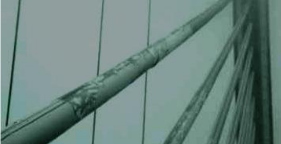
Ice on the stay cables of the VGCS bridge.
