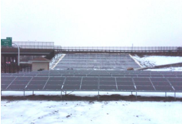
Solar arrays in the I-280 interchange at the north end of the VGCS bridge. Xunlight panels are mounted on a membrane on the overpass embankment ; First Solar panels are mounted on frames as shown in the foreground.
