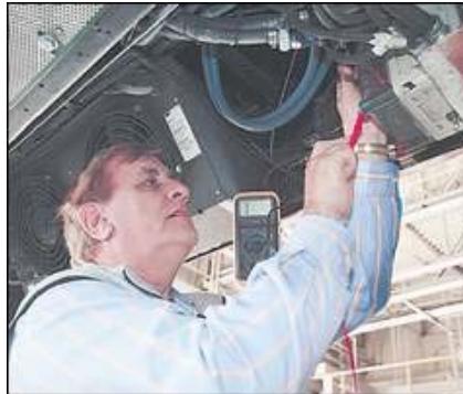
John Everton, president of H2 Engine Systems, checks controls under the modified minibus. The company is studying hydrogen-supplemented engine performance for TARTA.
